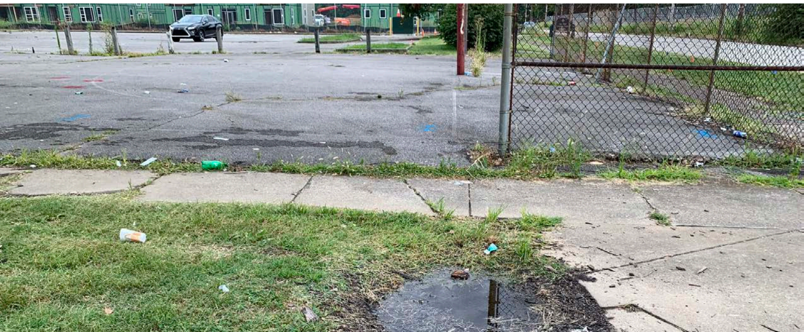
Deteriorated sidewalks and standing water at Baxter Square.
